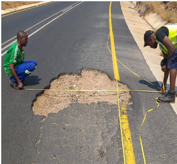
Pothole, crocodile cracking & pumping @ Km 30+000
