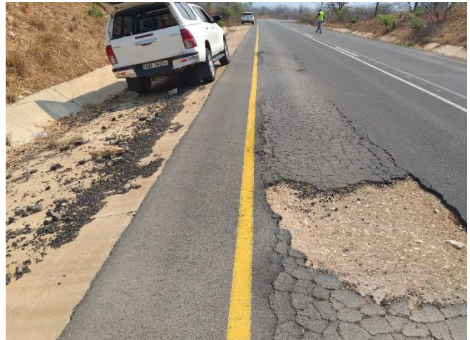
crocodile cracking, pumping & pothole @Km 25+700
