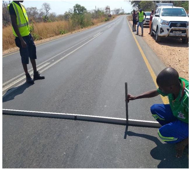
Bleeding &amp; rutting @ Km 72+400
