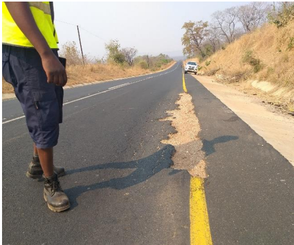
Shoving, crocodile cracking & potholes @Km 22+200
